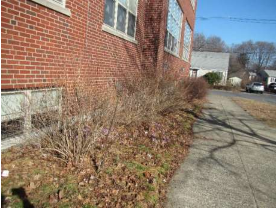
Bushes and trees near the building, including below univent air intakes
