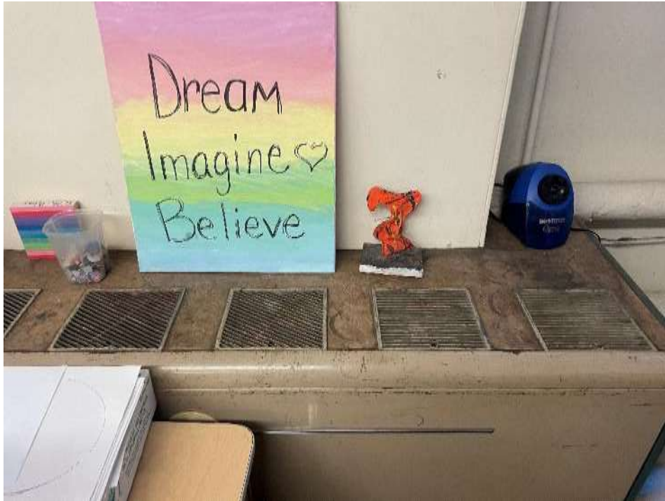
Top of a classroom univent, note furniture in front
